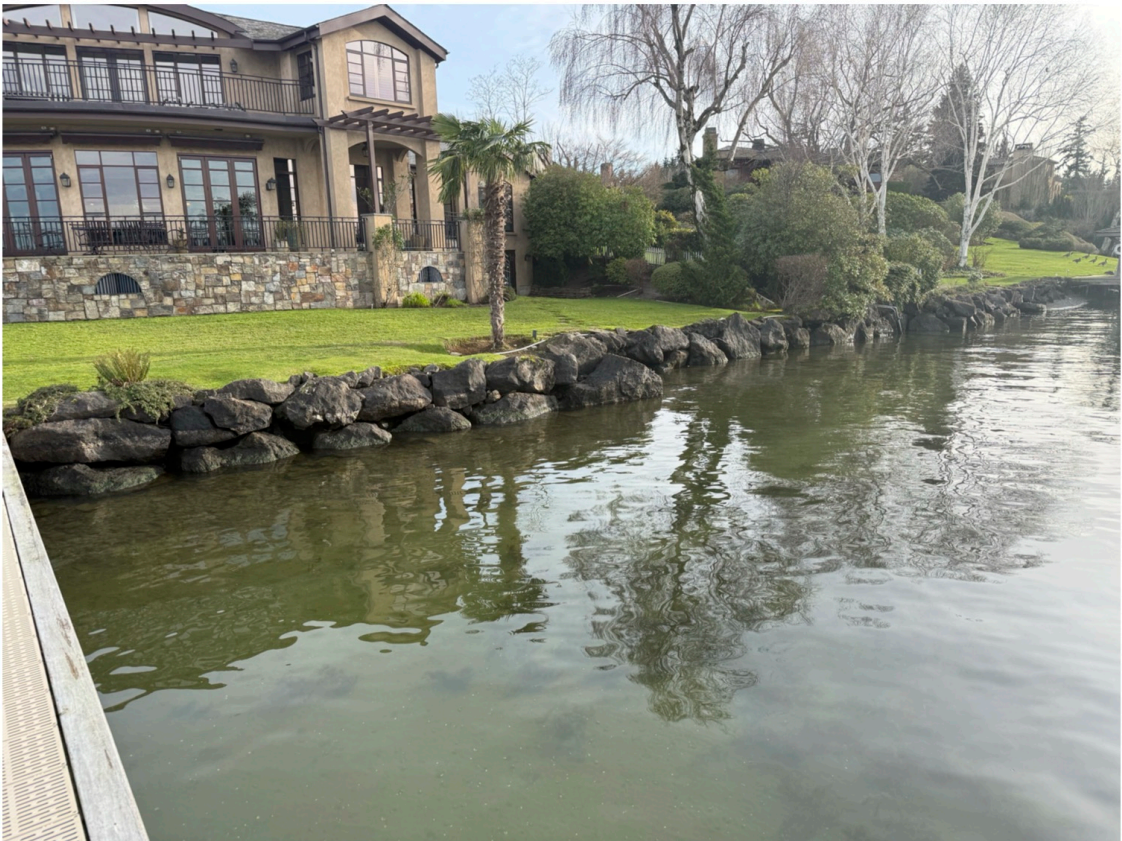
Photo 4 - Section of bulkhead to be repaired south of the dock.
